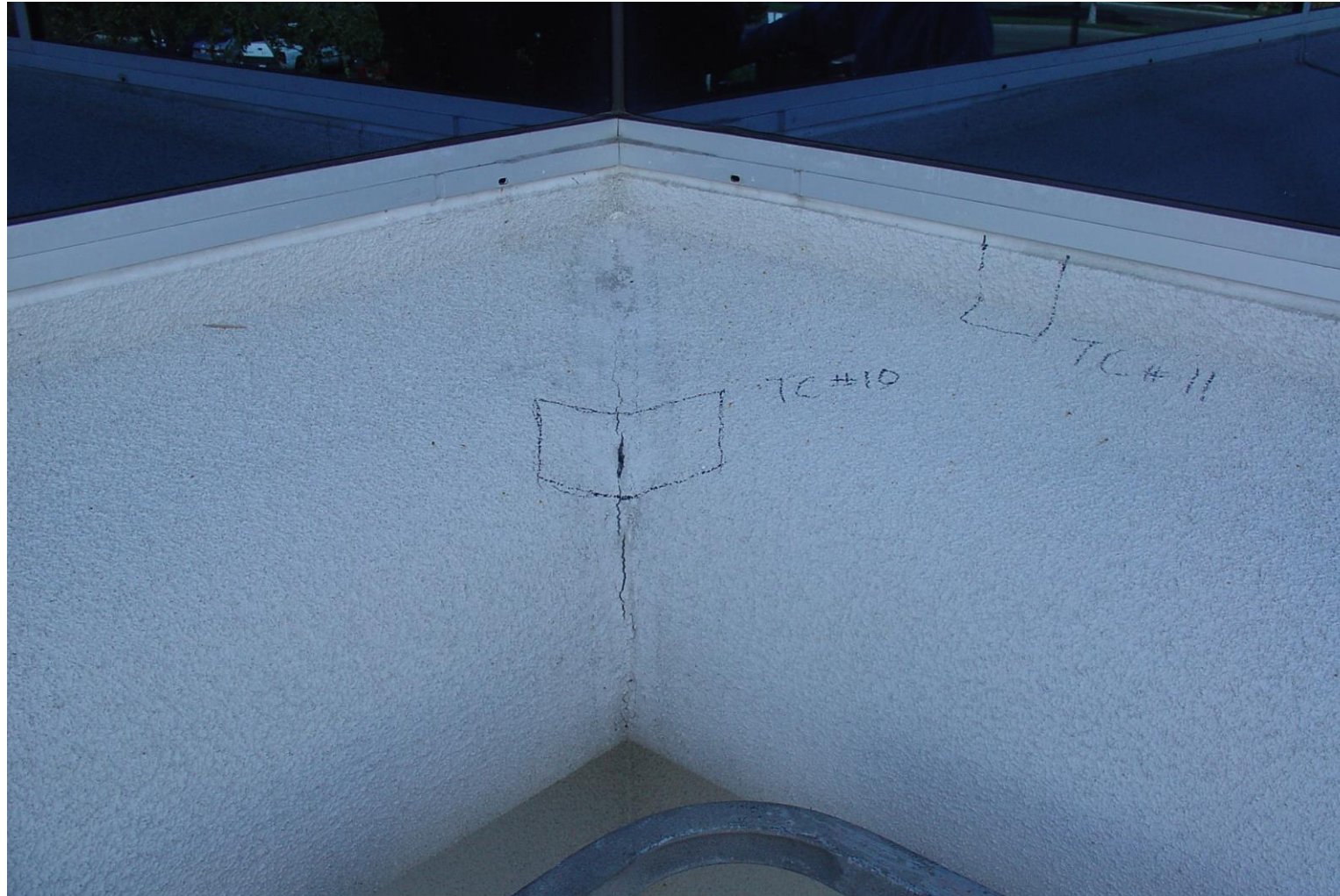
DEFECT: Lack of expansion joint at inside corners
