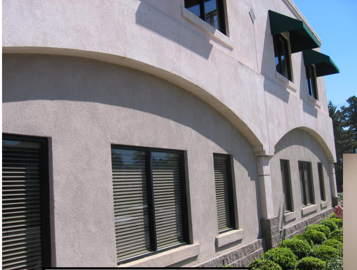
Few visible signs of distress
