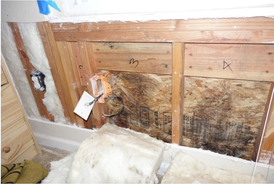
Figure 8: Uniform Damage Behind Fiber Cement Siding
