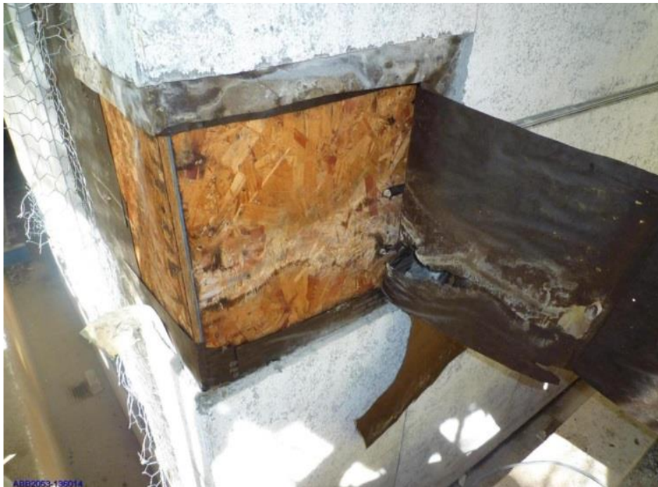
Figure 9B: Control Joint Impedes Water Drainage
