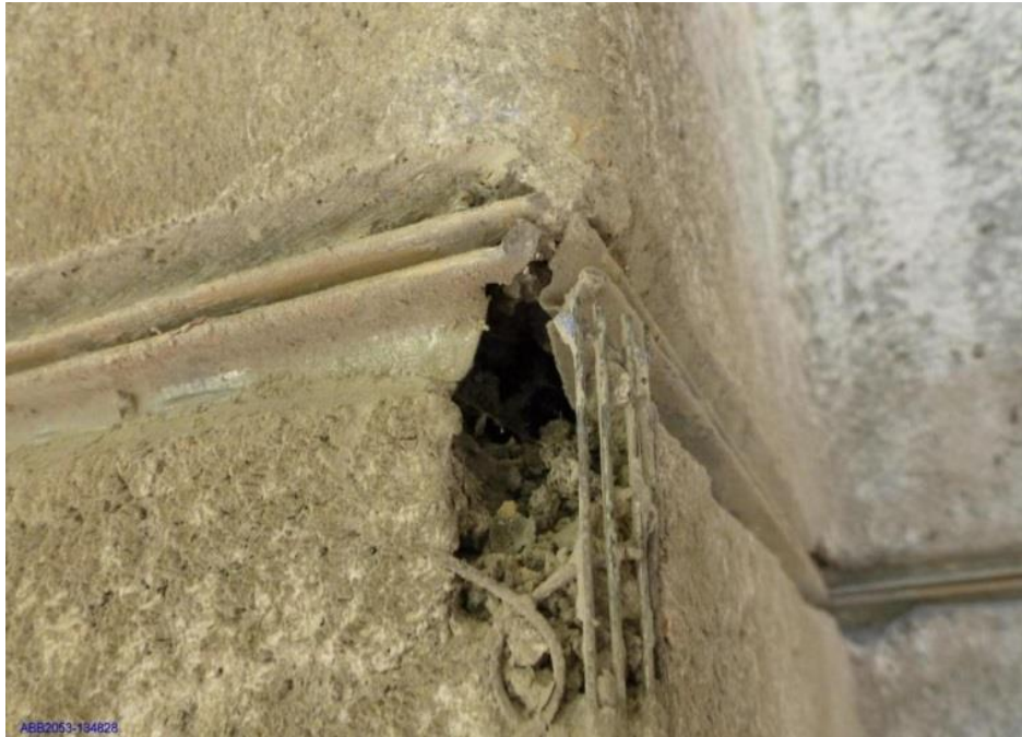
Figure 9A: Control Joint Corner Unsealed
