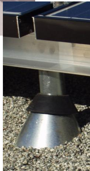
Figure 9. Penetrating roof mount on gravel ballasted BUR. The same detail would be applicable to an embedded-aggregate roof.
