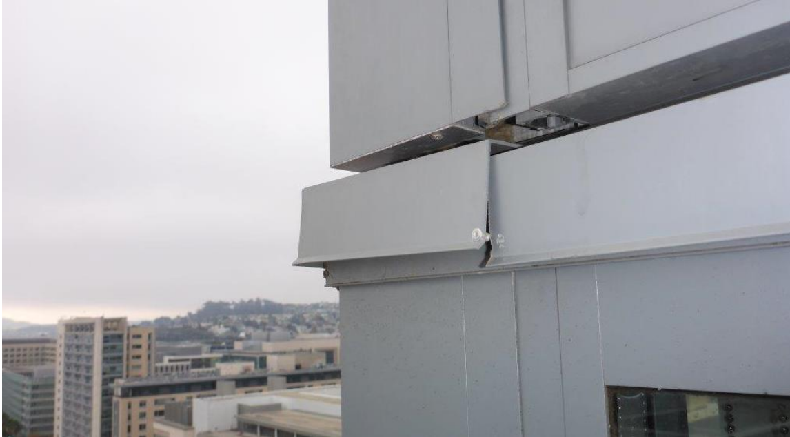
Figure 11: Sample of Trim Cover Failure
