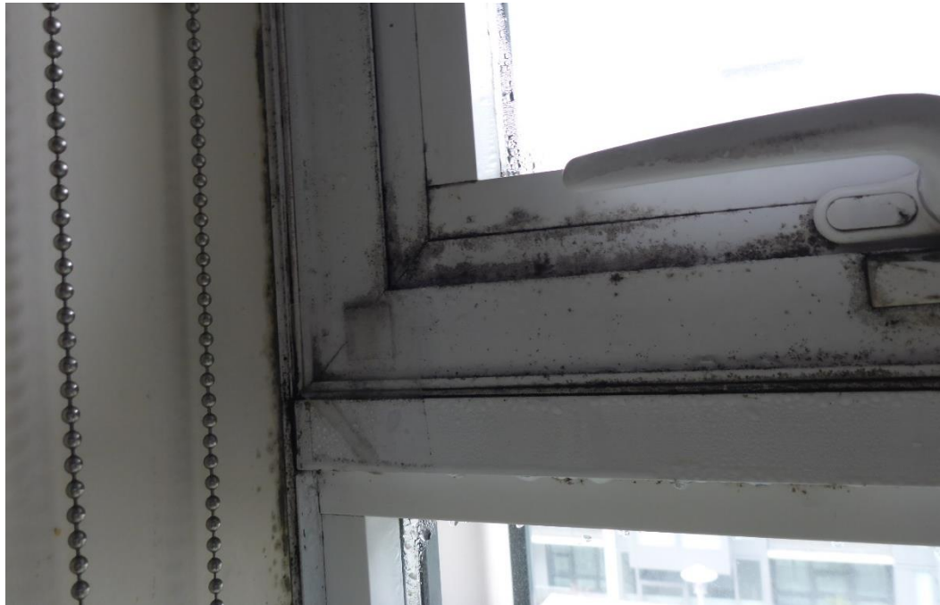
Figure 8: Example of Condensation Failure
