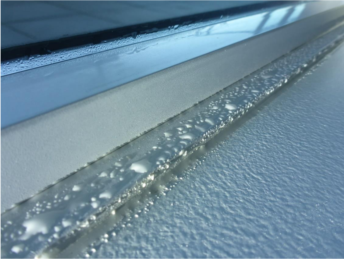
Figure 10: Condensation on an Interior Window Surface
