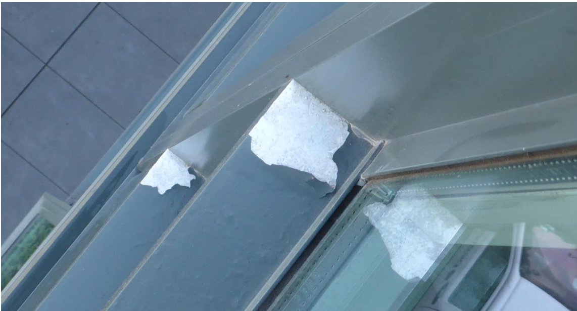
Figure 13: Example of Paint Failure
