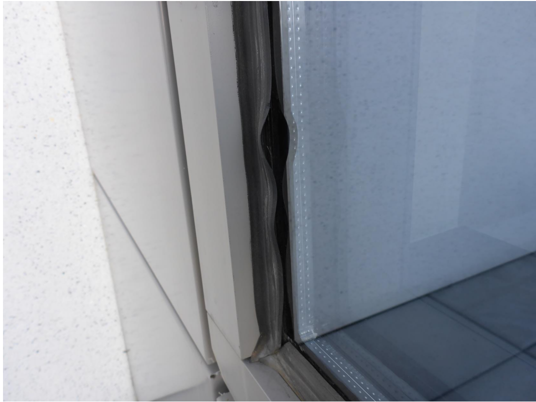
Figure 3: Example of Gasketing Failure
