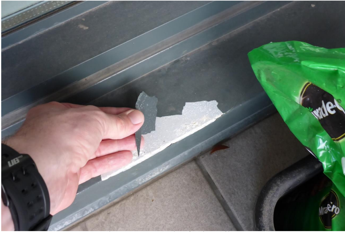
Figure 12: Example of Paint Failure
