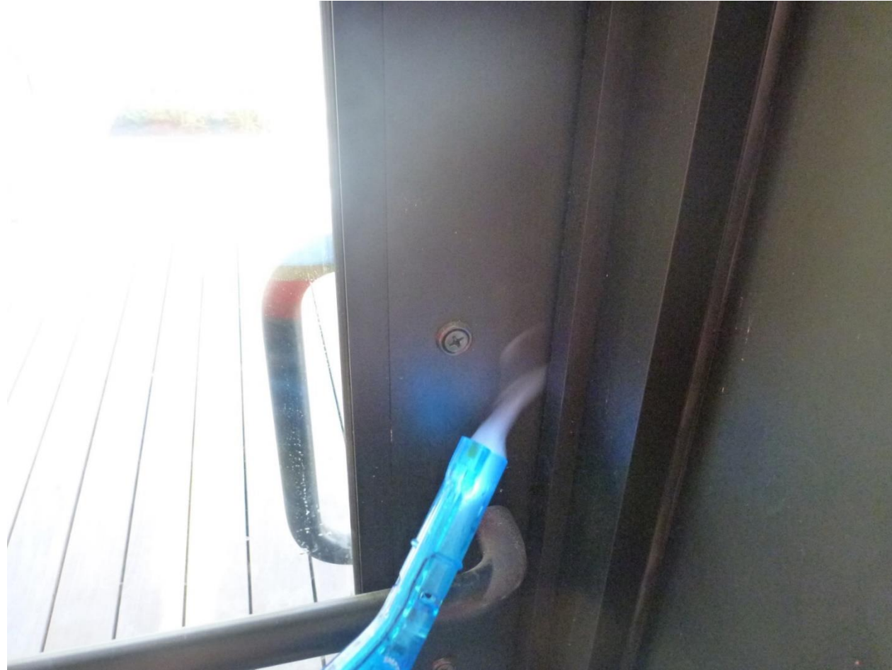
Air leakage identified by tracer testing
