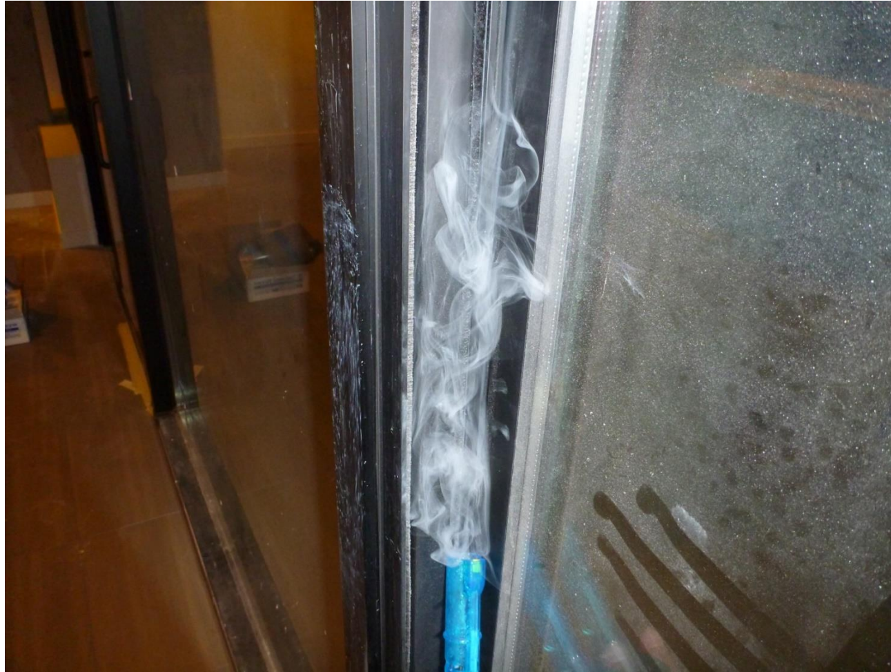
Tracer smoke test, no leakage
